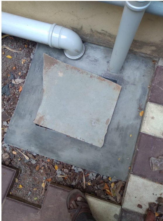
Rainwater collection tank for rain water harvesting
