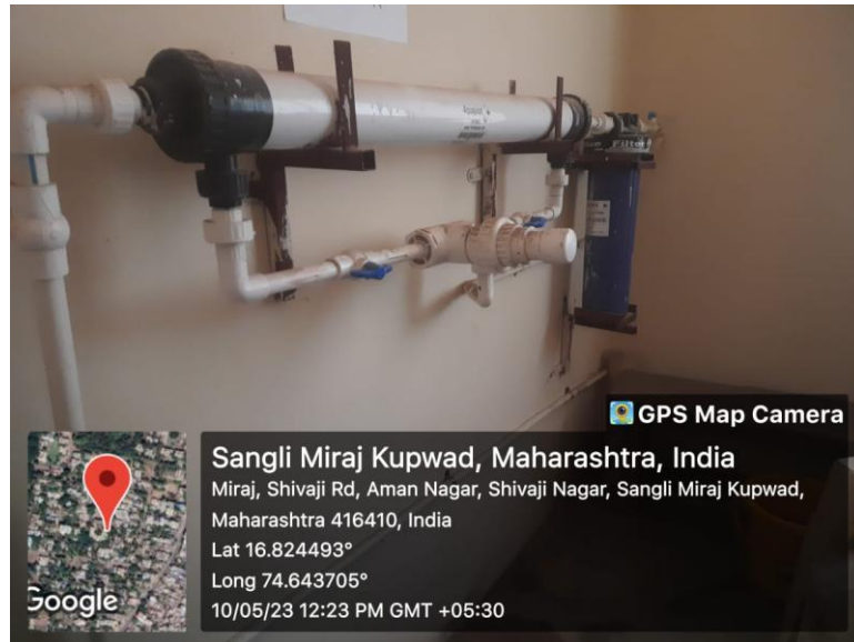
Advanced water filter unit
